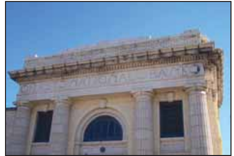
Appropriate Cornice Sign.
