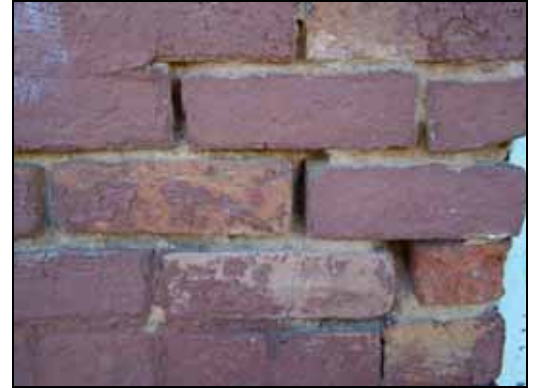
Crumbling mortar should be repointed.
