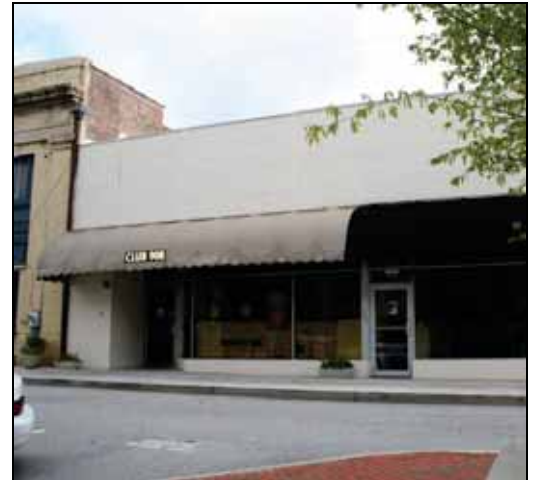
Inappropriate concave awning.
