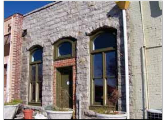
Inappropriate solid metal door.
