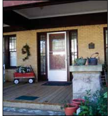
Inappropriate raw aluminum storm door.
