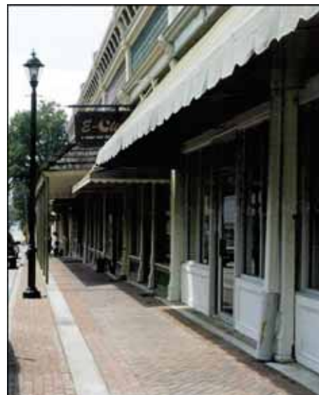
Inappropriate awning supported by sidewalk poles.
