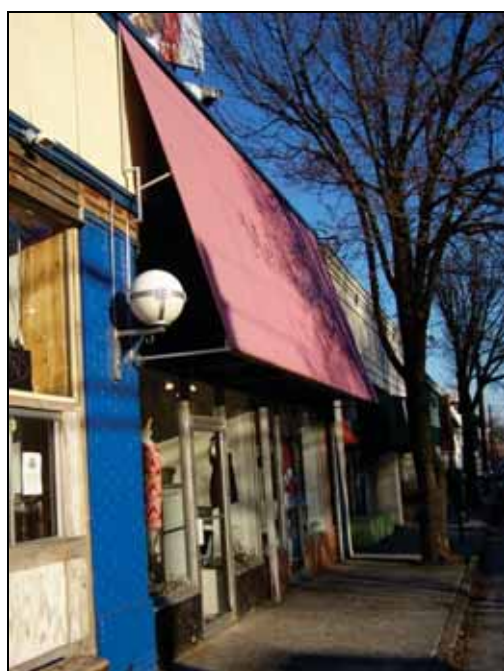
Inappropriately angled awning.
