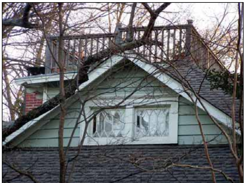
Inappropriate construction of a roof deck.
