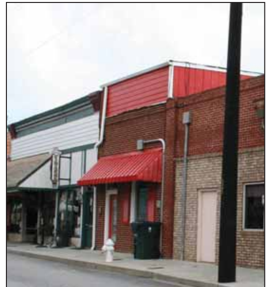
Inappropriate roof-top addition.
