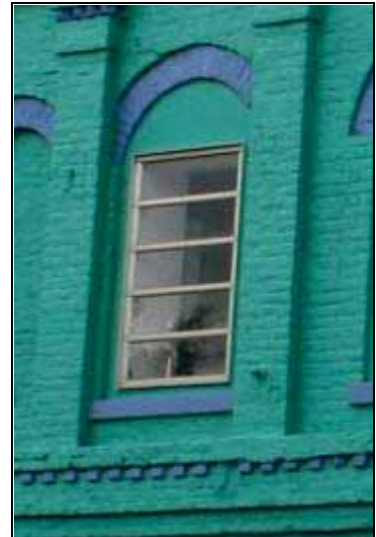
Inappropriate rectangular window in arched opening.
