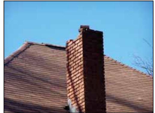
Inappropriate deterioration of a historic chimney.
