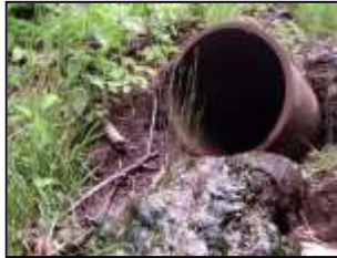
Ductile Iron Pipe (DIP)
