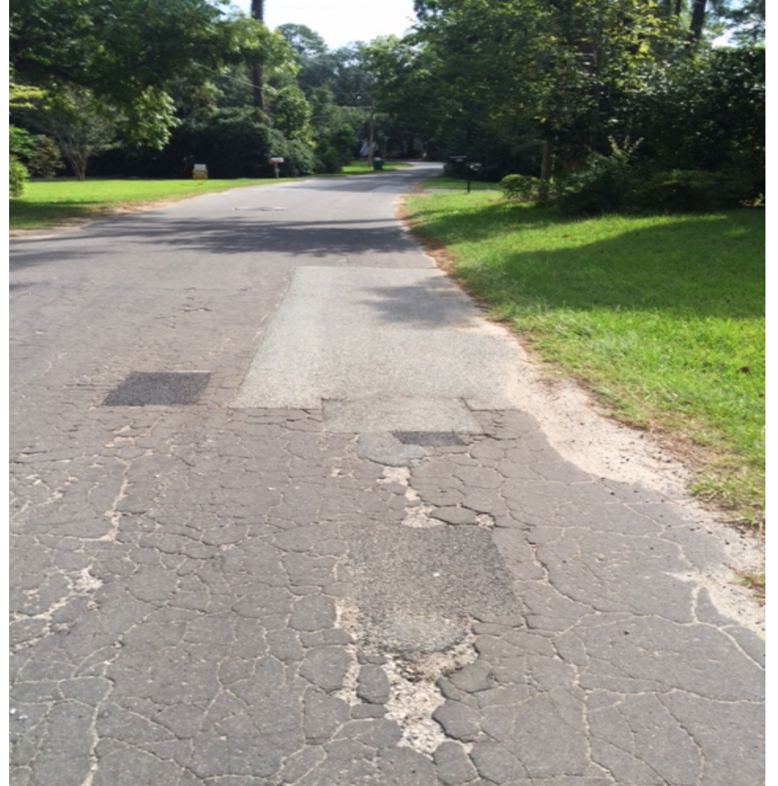
Patching or Potholes
