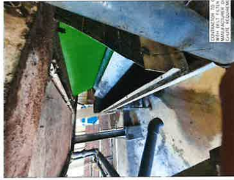
EXISTING DETERATERD SLUDGE DISCHARGE CONNECTION TO THE CONVEYOR
